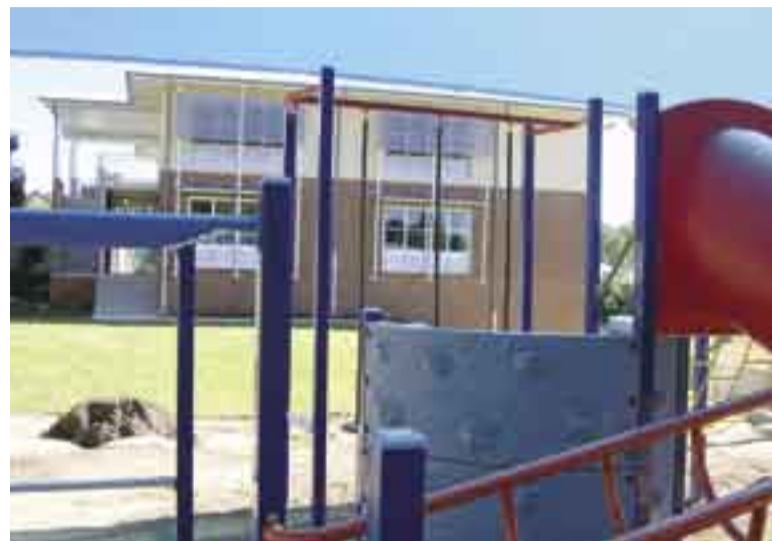
A new two-storey, four-classroom Prep building at Eatons Hill State School will have the school set for Prep in 2007.
