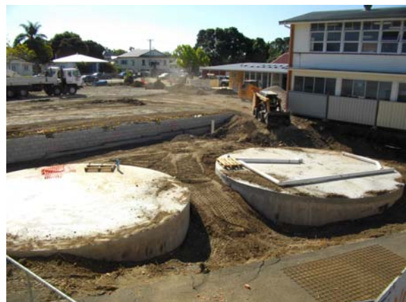
In ground water tanks
